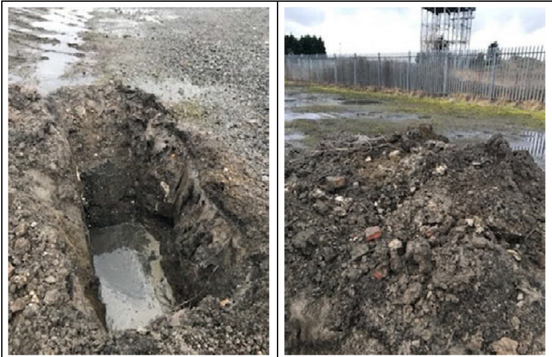
TP05 (Stone over geotextile, location is close to route of now culverted former deep and wide drain)
