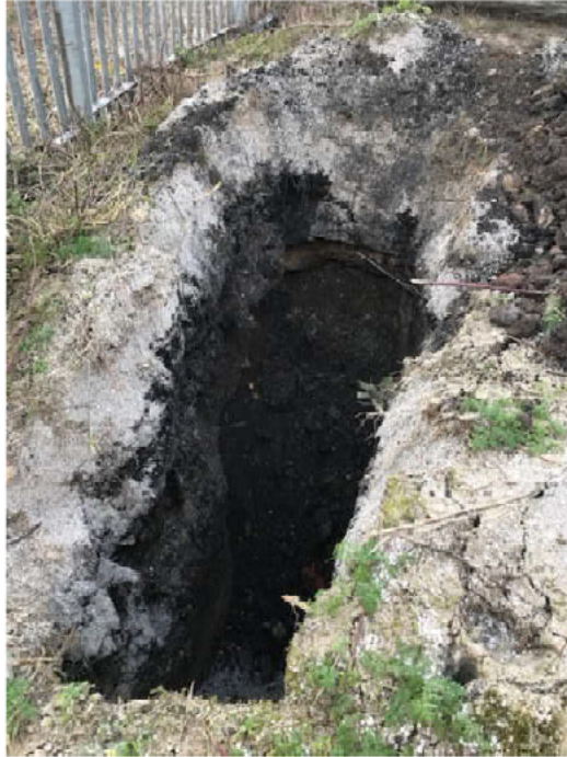
TP16 next to BH04 (Foundry sand waste, deep fill, Peat, possibly edge of backfilled culverted drain).
