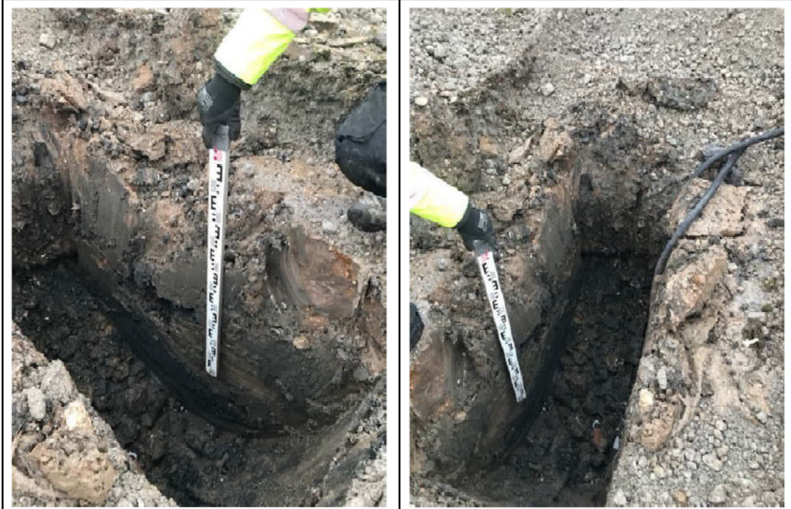
TP09 (Formation wet and contaminated, no CBR). Clay was of firm to stiff consistency). Most of area flooded in stone, water perched above clay fill or deeper where fill is granular.
